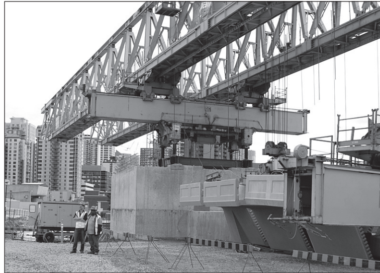
From left: crews have already excavated 220,000 cubic metres and dug 12 metres deep for the future underground Westbrook Station; the launching truss began lifting sections of the elevated track at Shaw Millennium Park last month.
